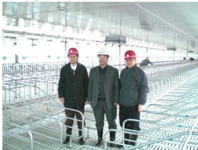
Above: A building in the 2,500-sow farm unit under construction near central Henan Province, where Shineway is currently adding a modern 10,000-sow production base
